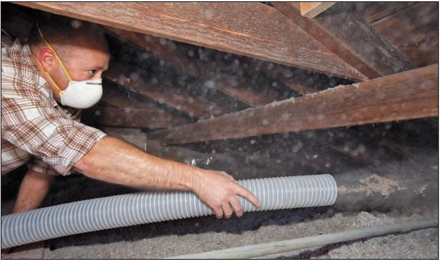
Wes Harding, owner of Harding Construction & Sustainable Solutions, installs cellulose insulation in an attic at a home in Naples. Cellulose insulation contains more than 80 percent recycled content and is more effective than conventional insulation. (Photograph by the Business Journal's Thomas McConville)
