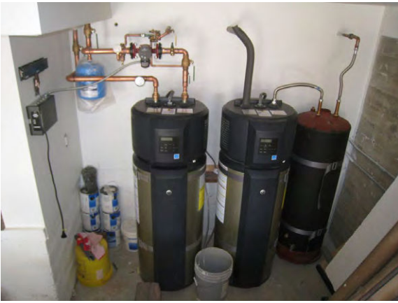
Water tanks in the passively heated garage
