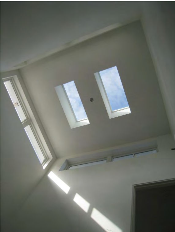
Thermal chimney's ventilating skylights
