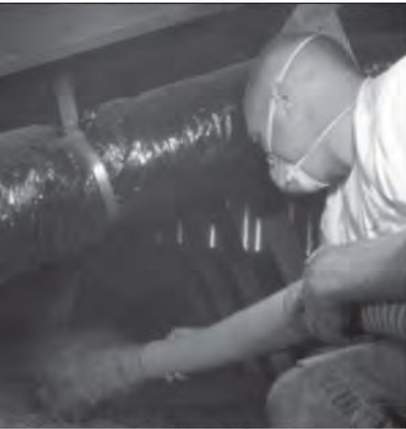
ion into cracks and crevices. A dirty job, but somebody's got to do it.
